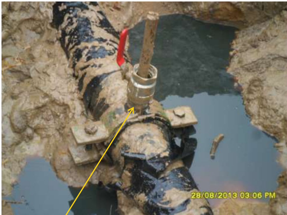
Close up: Illegal fitting on 6" Obigbo North-Ogale pipeline at Ogale. Picture was taken during Joint Investigation of 28 th August 2013.
