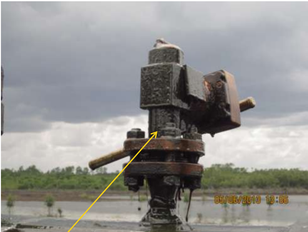
Close up : Tampered valve on 28" old Nembe Creek pipeline riser at Ido. Picture was taken during Joint Investigation of 5 th June 2013.
