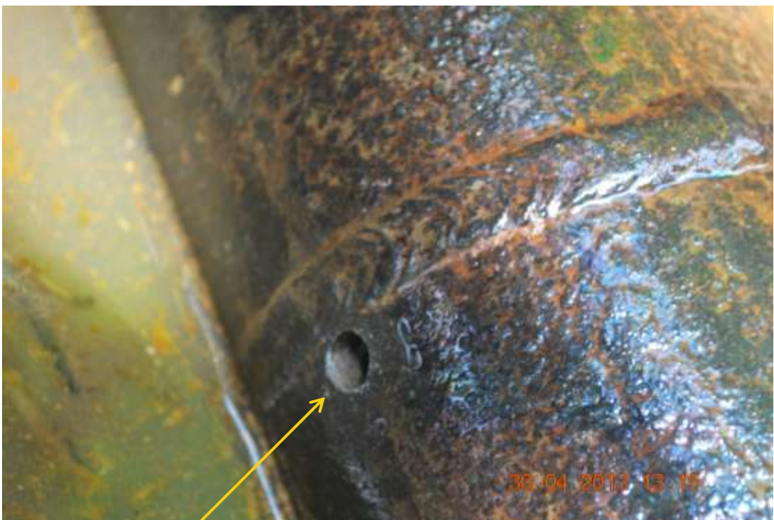
Close up: Drilled hole on Adibawa Well2S flowline at Edagberi. Picture was taken during Joint Investigation of 30 th April 2013.
