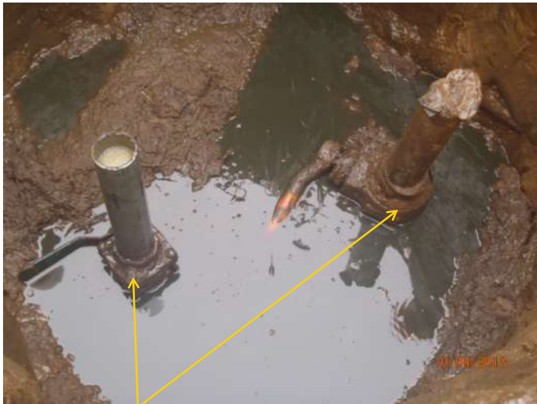
Close up: Illegal fittings on 12" Oguta-Egbema pipeline at Opuoma-Oguta. Picture was taken during Joint Investigation of 10 th April 2013.
