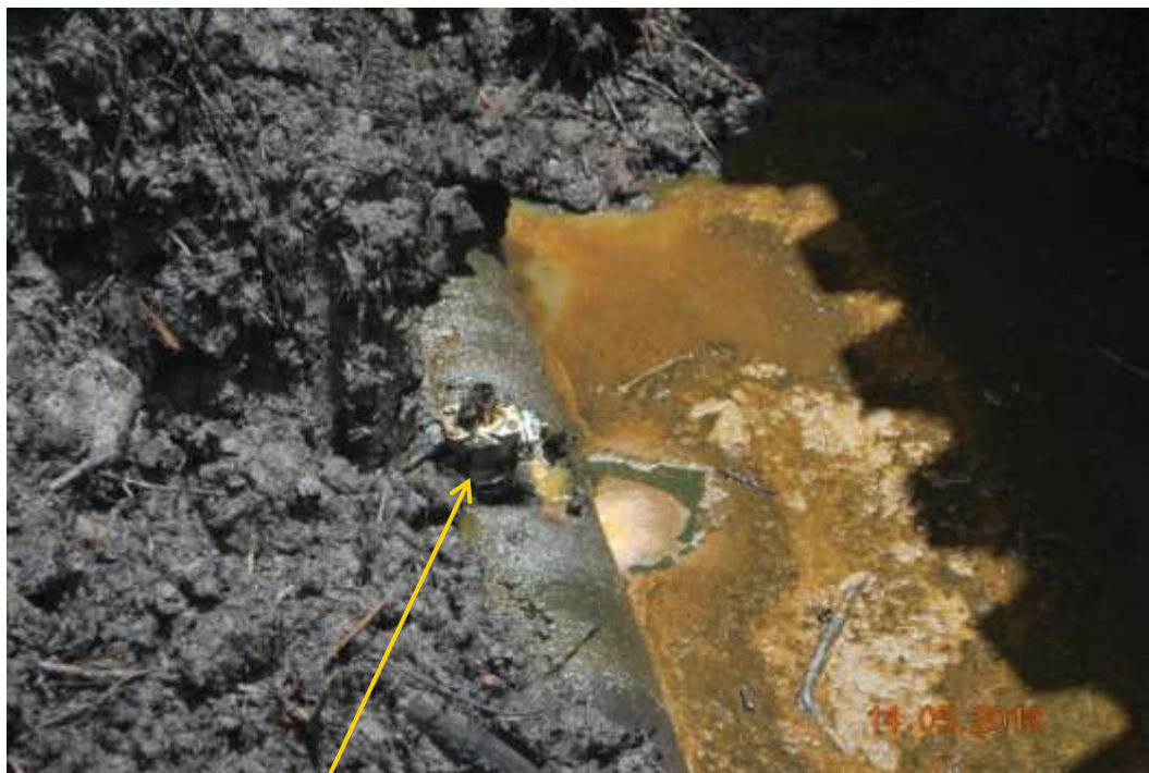
Close up: Illegal fitting on 20" Opukushi-Brass Creek trunkline at Tamogbene. Picture was taken during Joint Investigation of 14 th May 2013.
