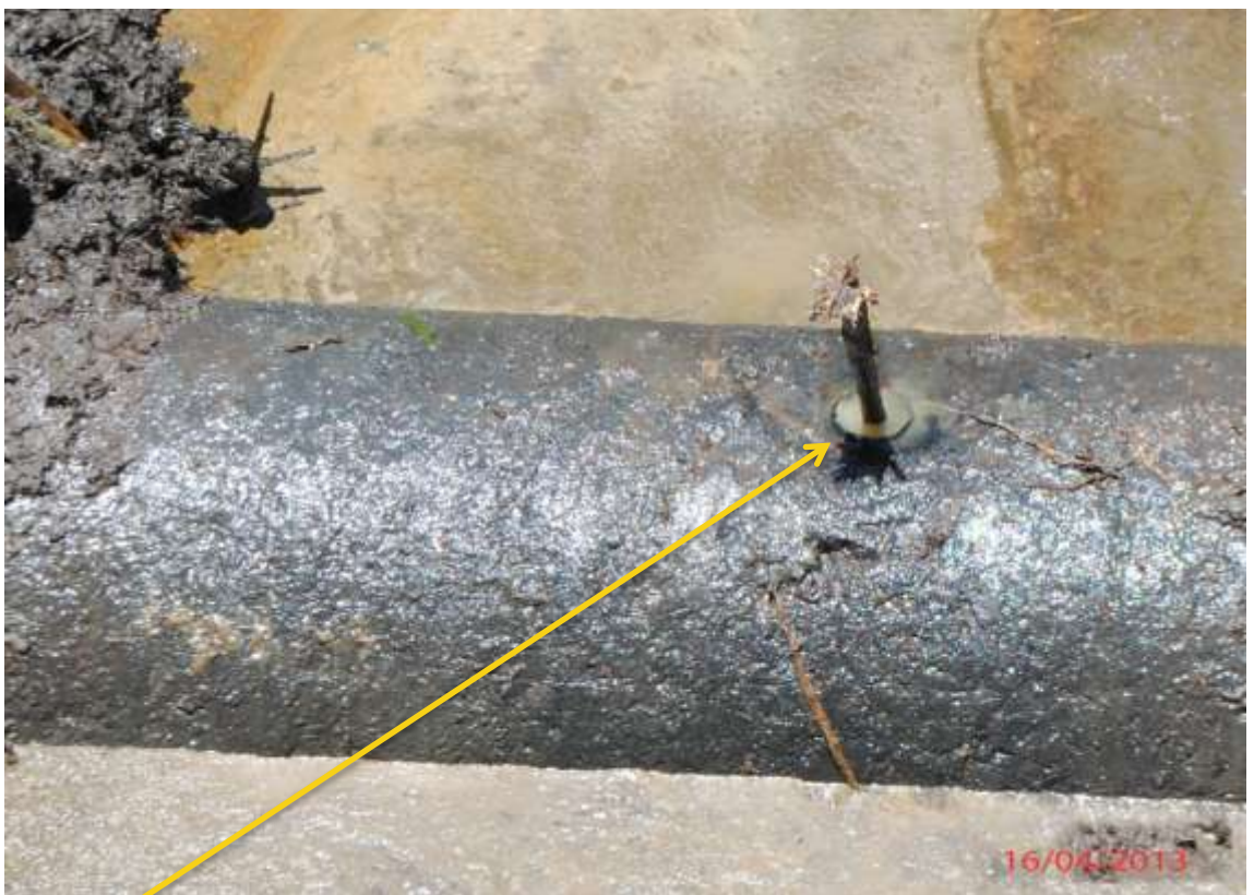
Close up: Illegal fittings on 20" Opukushi - Brass Creek Pipeline at Tamogbene. Picture was taken during Joint Investigation of 16 th April 2013.
