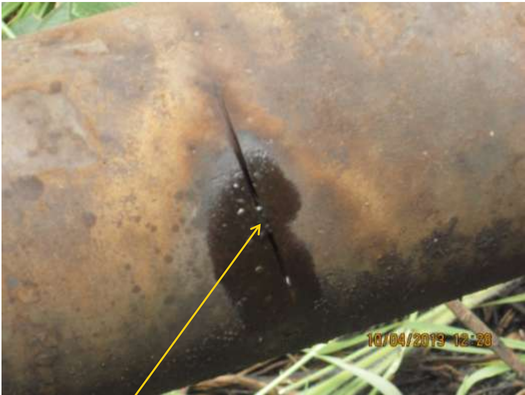
Close up: Hacksaw cut on 4" Adibawa Well10S flowline at Edagberi. Picture was taken during Joint Investigation of 10 th April 2013.
