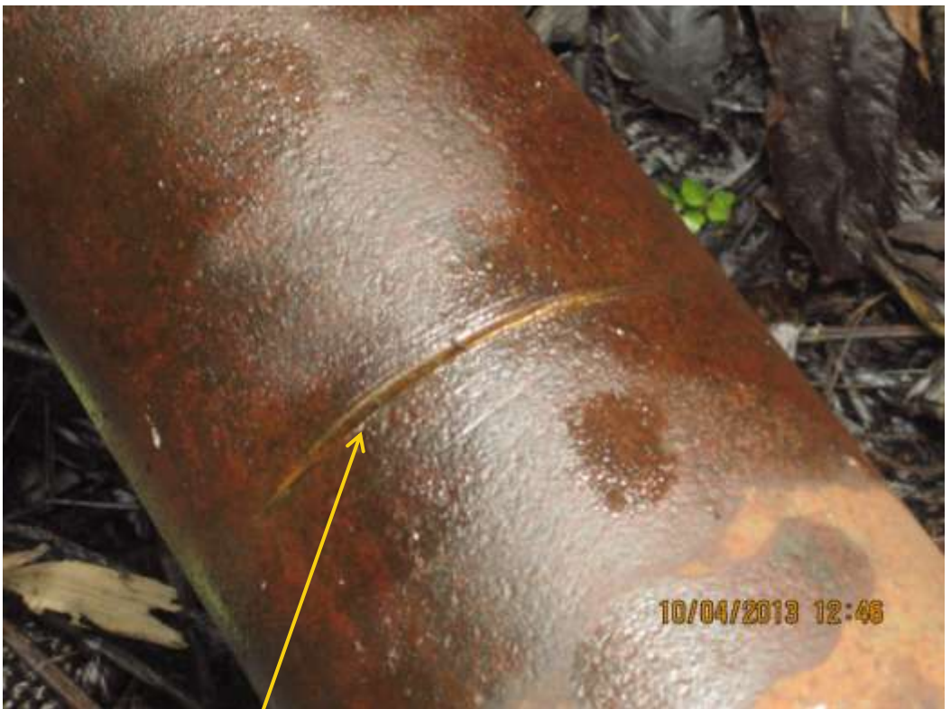
Closeup: Hacksaw cut on 4" Adibawa Well10S flowline at Edagberi. Picture was taken during Joint Investigation of 10 th April 2013.
