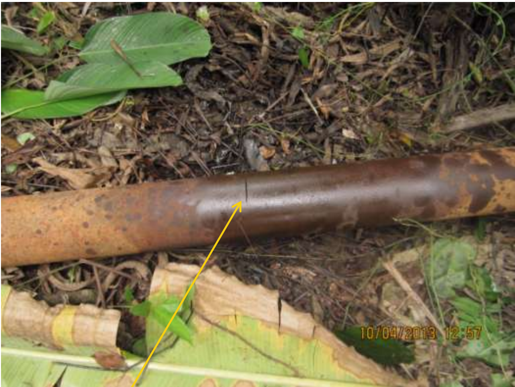
Close up: Hacksaw cut on 4" Adibawa Well10S flowline at Edagberi. Picture was taken during Joint Investigation of 10 th April 2013.
