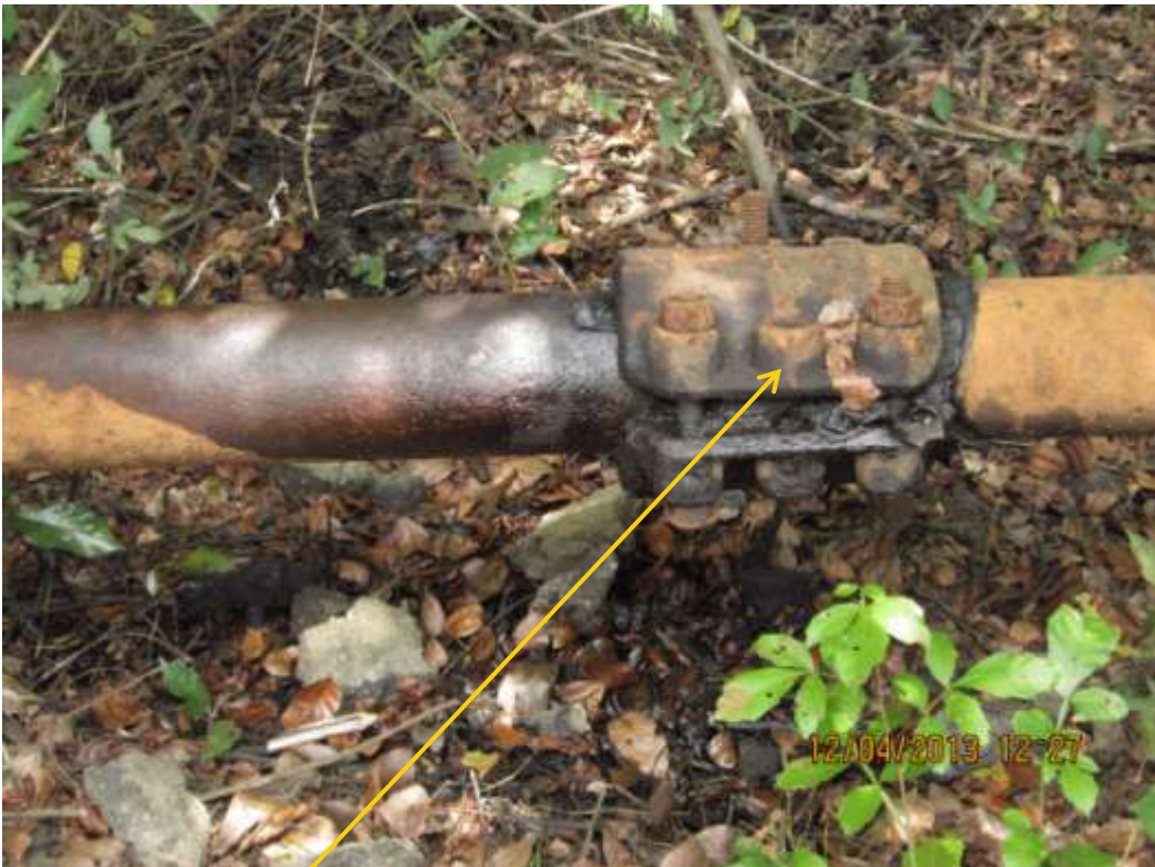
Close up: Location of missing bolt and nut on 4" Adibawa Well8S flowline at Edagberi. Picture was taken during Joint Investigation of 12 th April 2013.
