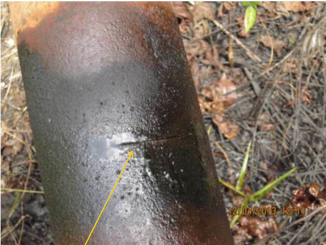
Close up: Hacksaw cut on 4" Adibawa Well8S flowline at Edagberi. Picture was taken during Joint Investigation of 12 th April 2013.
