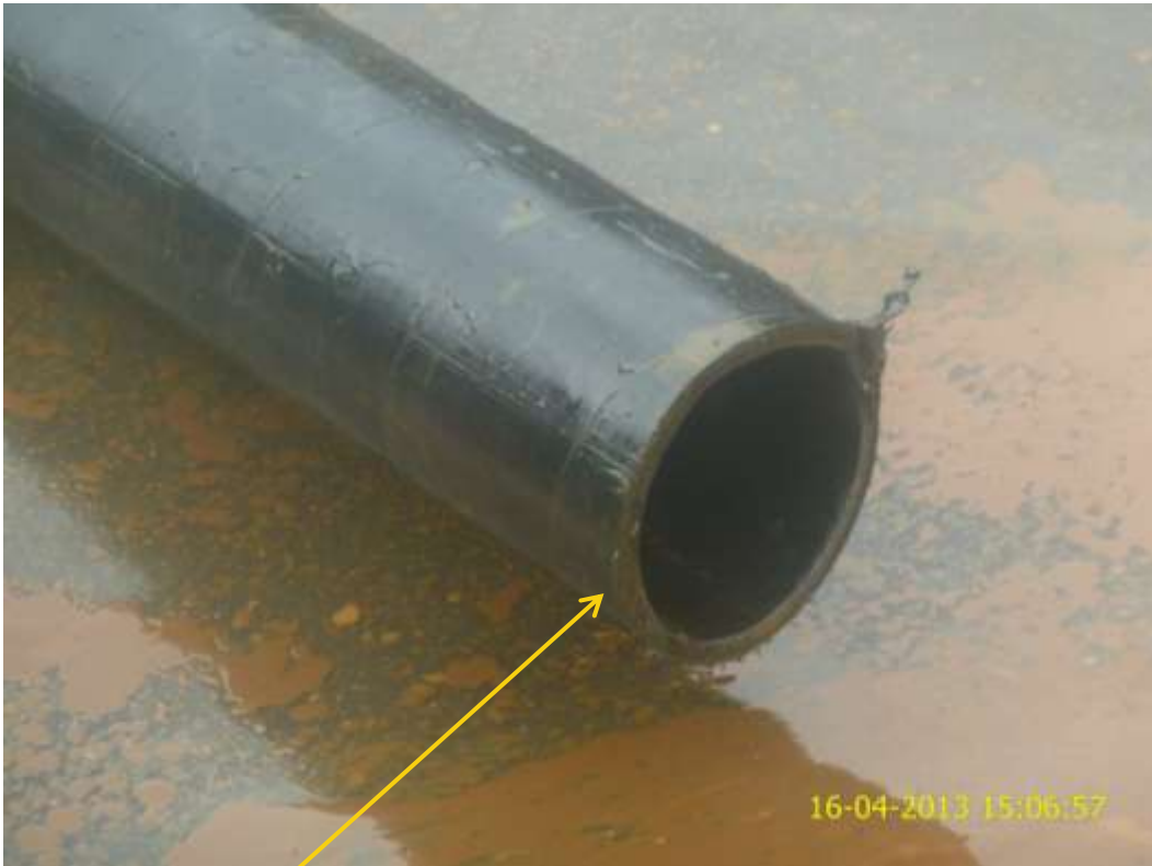
Close up: Cut section on Nembe1 Well23T flowline at Ewesuo. Picture was taken during Joint Investigation of 16 th April 2013.
