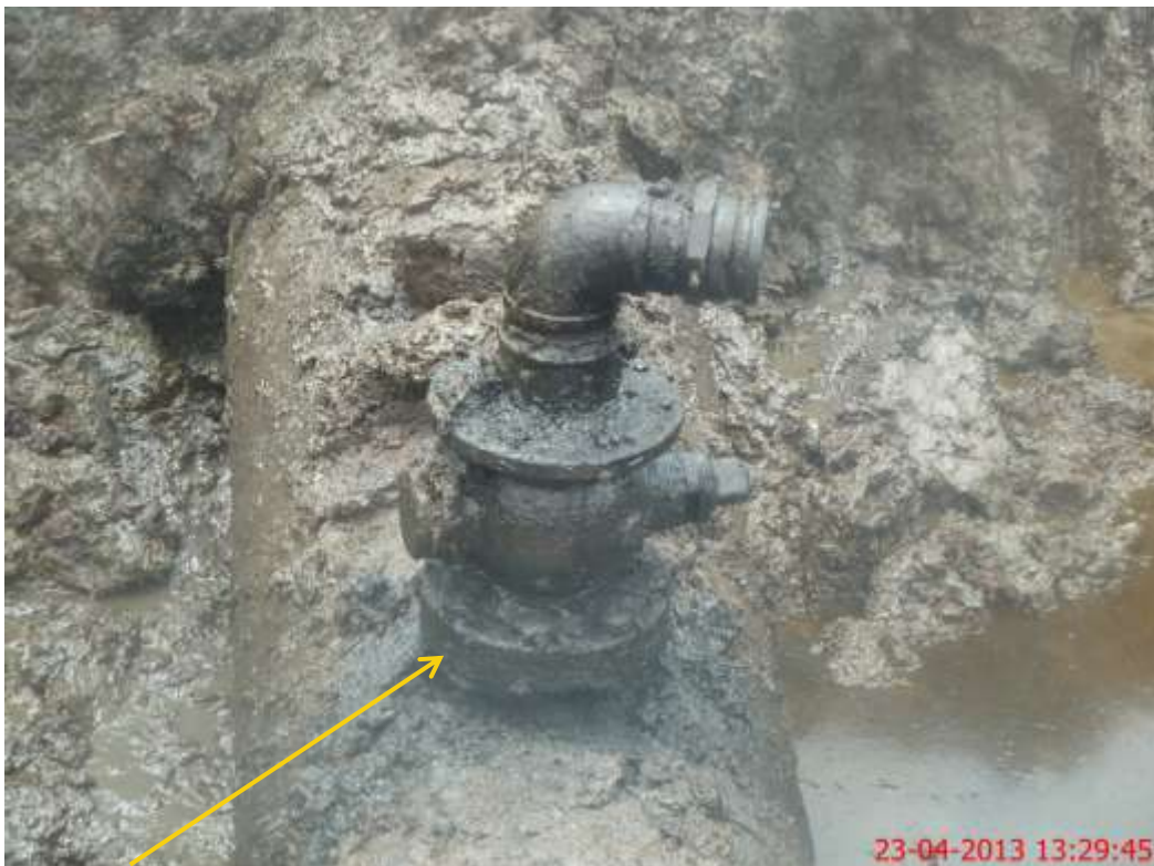
Close up: Bunkering Fitting on 24" Bomu-Bonny Trans Niger Pipeline at Bodo City. Picture was taken during Joint Investigation of 23rd April 2013.
