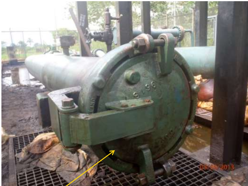
Close up: Leaking barrel door at Assa manifold. Picture was taken during Joint Investigation of 3 rd May 2013.
