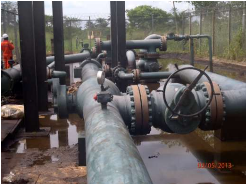
Overview: Part of spill impact at Assa manifold. Picture was taken during Joint Investigation of 3 rd May 2013.
