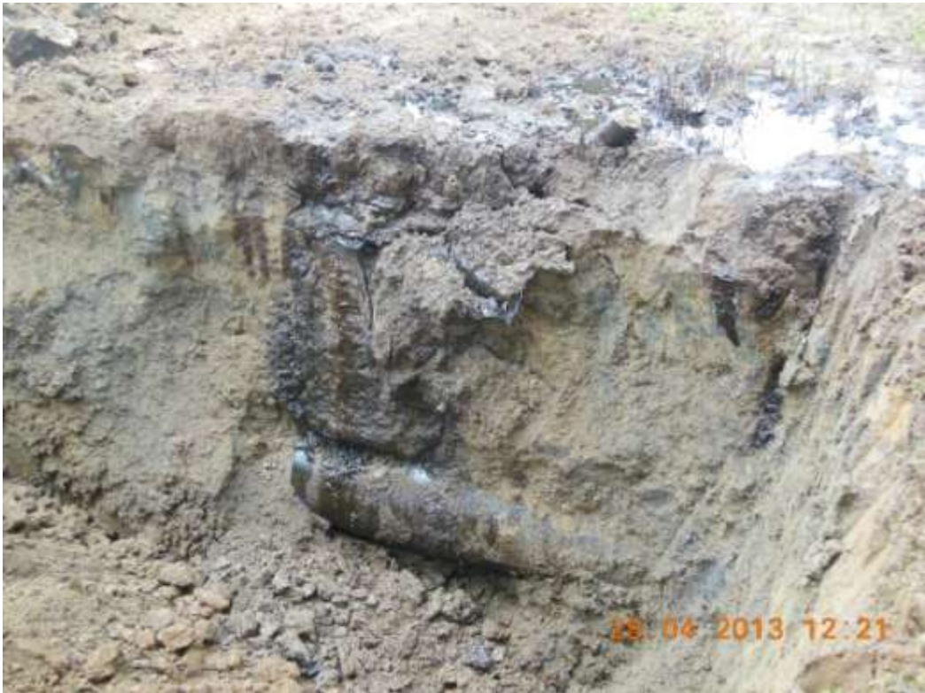
Overview: Part of spill impact on 24" Nkpoku-Bomu Trans Niger pipeline at Eelenwo. Picture was taken during Joint Investigation of 28 th April 2013.
