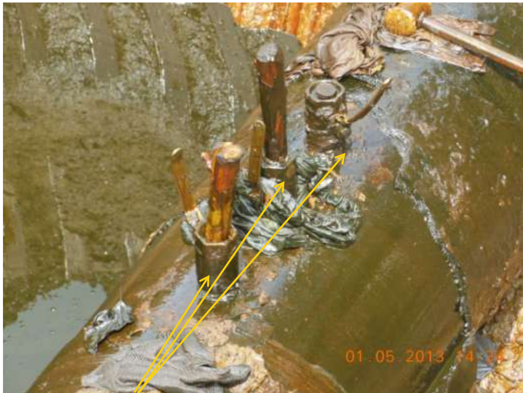
Close up: Illegal fittings on 24" Nkpoku-Bomu Trans Niger pipeline at Eelenwo. Picture was taken during Joint Investigation of 1 st May 2013.
