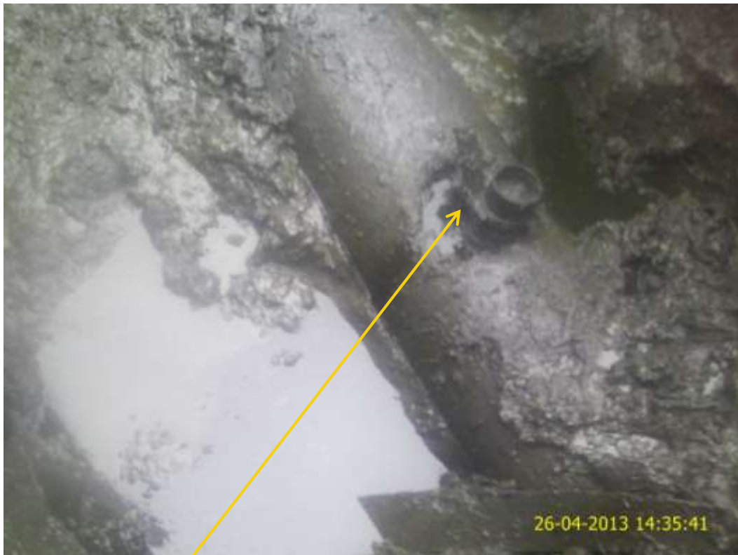
Close up: Illegal fitting on 24" NembeCreek pipeline at Kalibiama. Picture was taken during Joint Investigation of 26 th April 2013.
