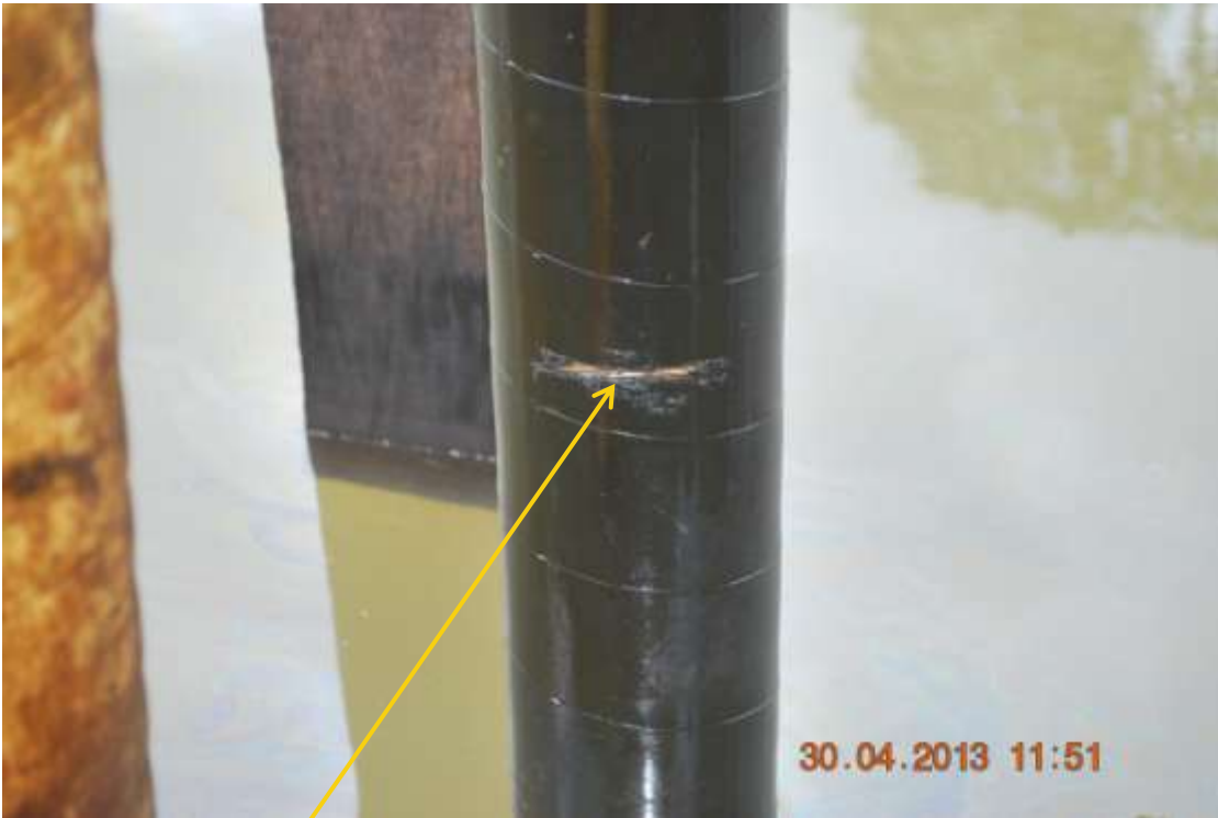
Close up: Illegal fittings on Benisede Well 11 flowline at Amabulou. Picture was taken during Joint Investigation of 30 th April 2013.
