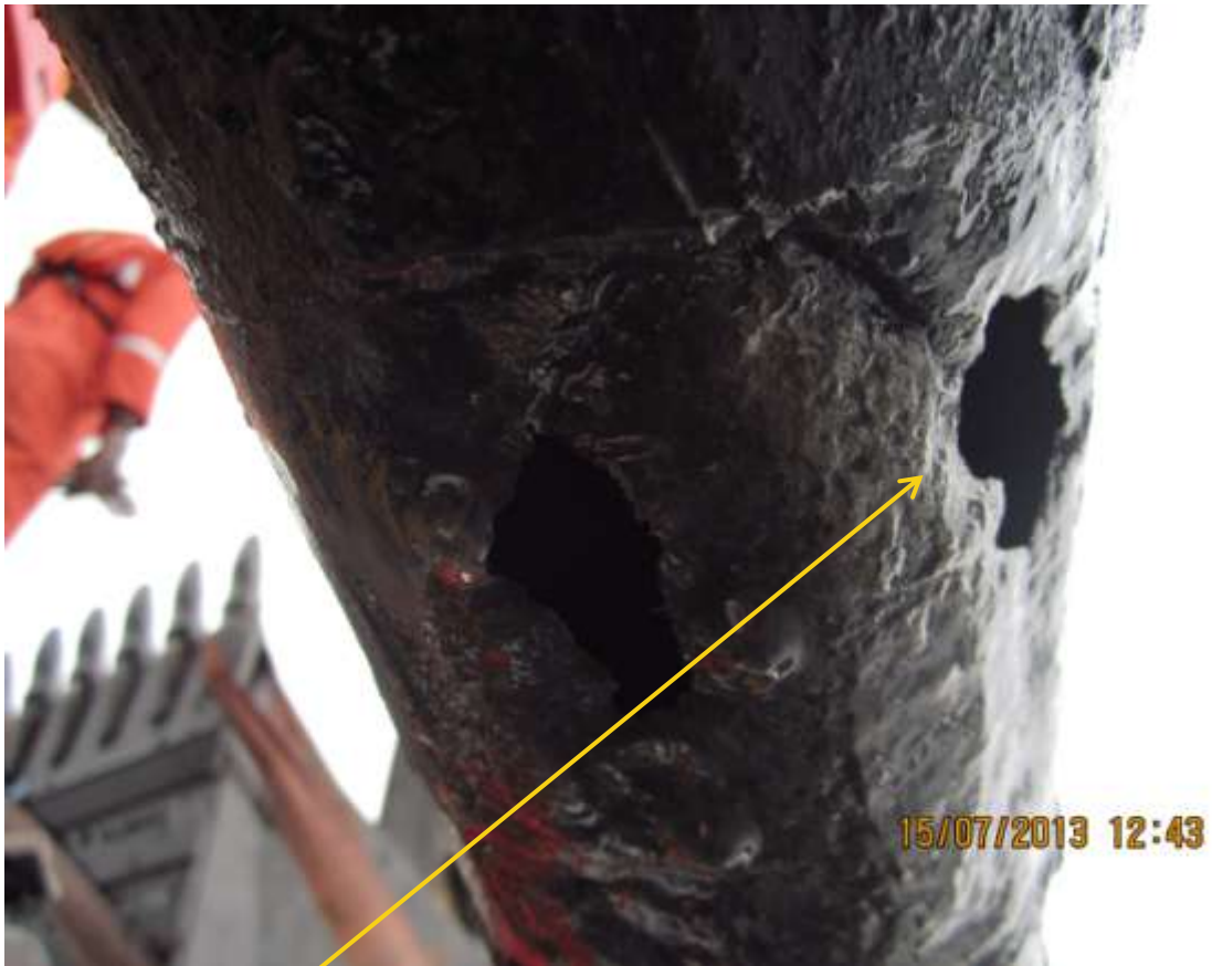
Close up : Spill due to corrosion on Bonny Well2S flowline at Oloma. Picture was taken during Joint Investigation of 15 th September 2013.
