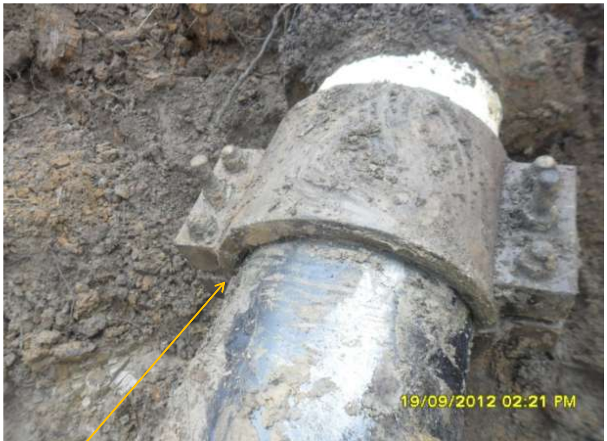
Close-up: Failed clamp on 18" Assa - Rumuekpe Trunkline at Awara. Picture was taken during Joint Investigation of 19 th Sept. 2012..
