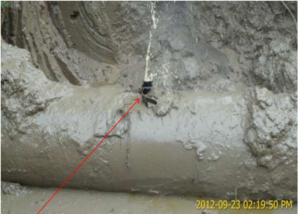
Close-up: Illegal fitting on 20'' Buguma-Alakiri Trunkline at Daily Bread (Bukuma). Picture was taken during Joint Investigation of 23 rd Sept. 2012.
