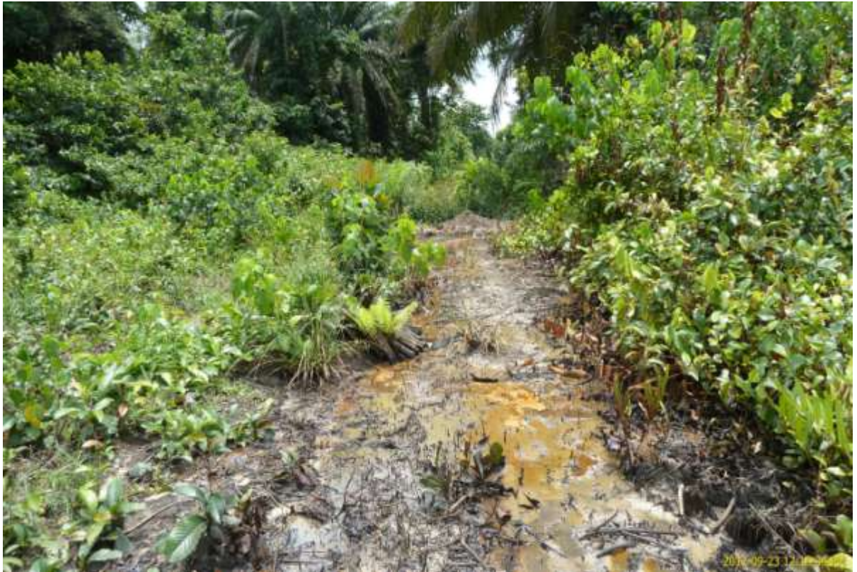
Overview: Part of spill impact on 20'' Buguma-Alakiri Trunkline at Daily Bread (Bukuma). Picture was taken during Joint Investigation of 23 rd Sept. 2012.
