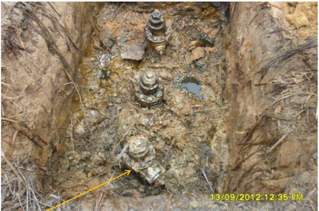
Close-up: Illegal fittings on 16'' Uzere-Eriemu Pipeline at Iyede. Picture was taken during Joint Investigation of 13 th Sept. 2012.
