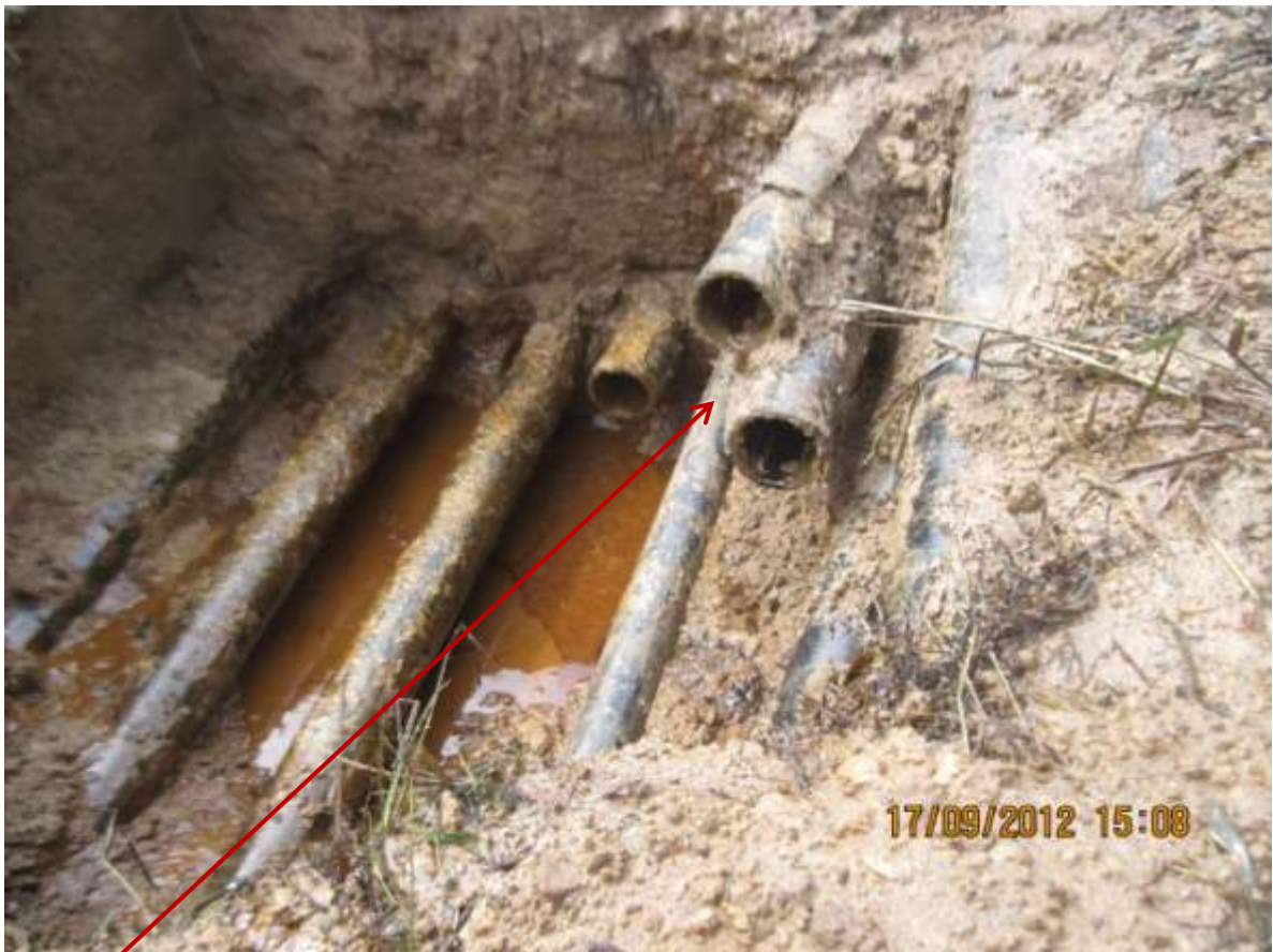
Close-up: Missing flowlines from Agbada 2 Well 41, 42 and 43 flowlines at Umuohia. Picture was taken during Joint Investigation of 17th Sept. 2012.
