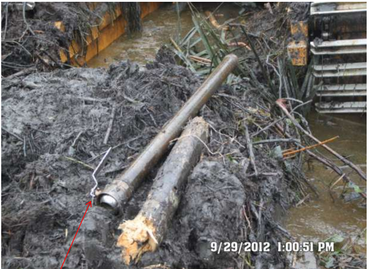
Close-up: Illegal fitting on 20" Opukushi-Brass Creek Trunkline at Opukushi. Picture was taken during Joint Investigation of 29 th Sept. 2012.
