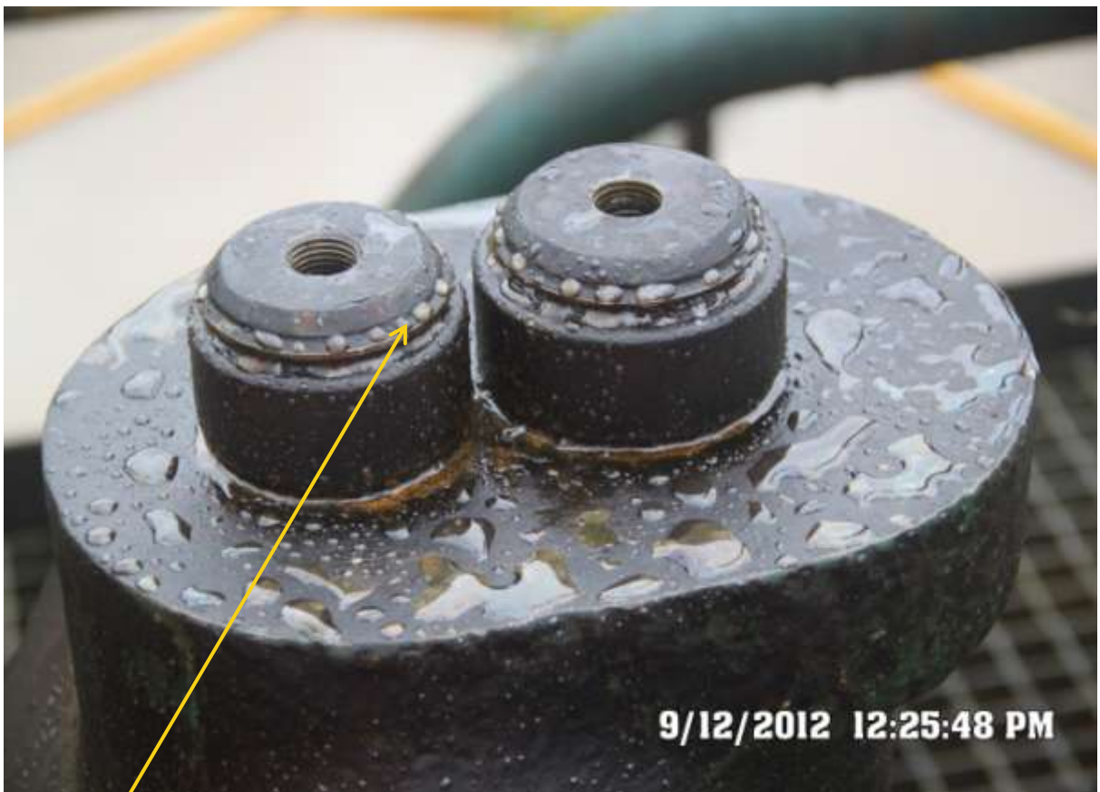
Close-up: Illegal Wellhead tampering on Benisede Well 15T at Ojobo. Picture was taken during Joint Investigation of 12th Sept. 2012.
