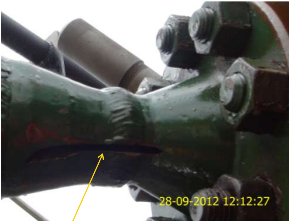
Close up: Deep cut on Nembe Creek1 Well19S wellhead at Mile1. Picture was taken during Joint Investigation of 28 th September 2012.
