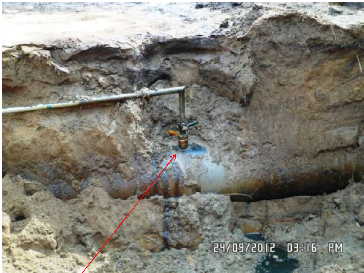
Close-up: Illegal fitting on 28" Nkpoku - Bomu Pipeline at Gio. Picture was taken during Joint Investigation of 24 th Sept. 2012.
