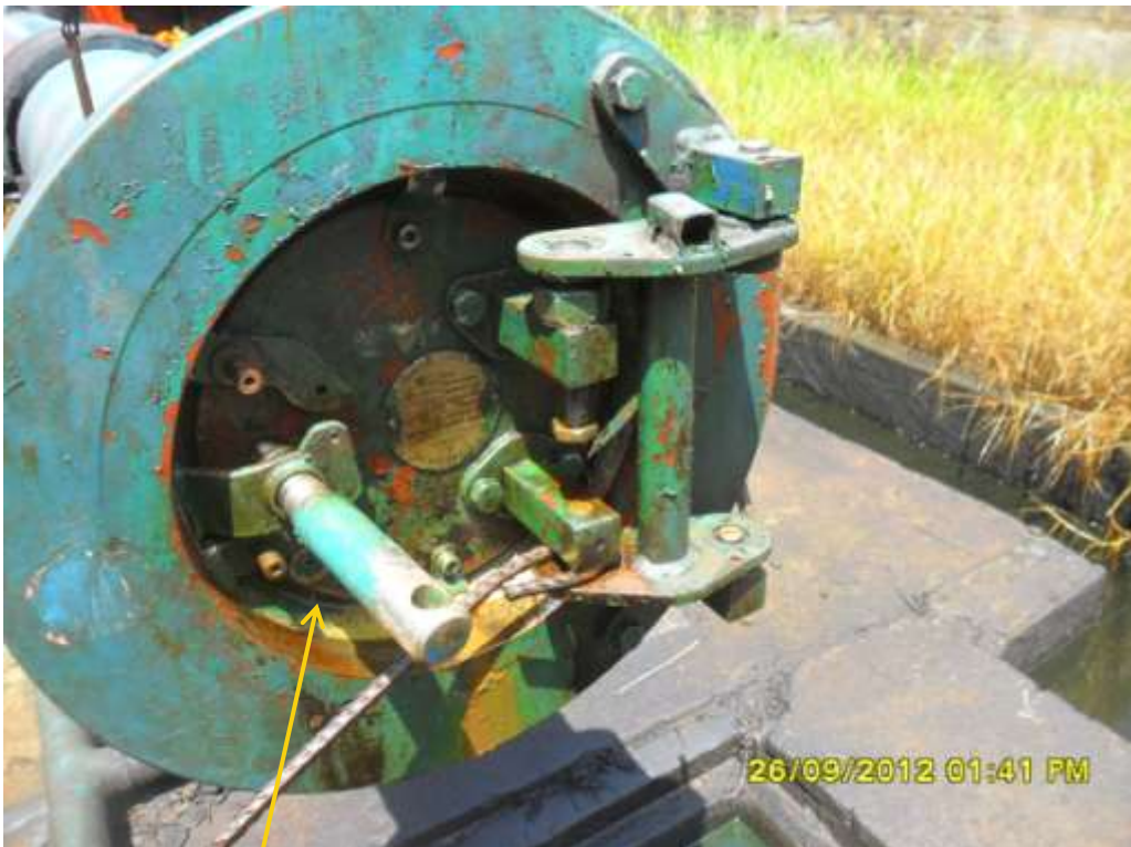
Close up: Leak from barrel door on 8" Ubie pipeline manifold at Ukpeliède. Picture was taken during Joint Investigation of 26 th October 2012.
