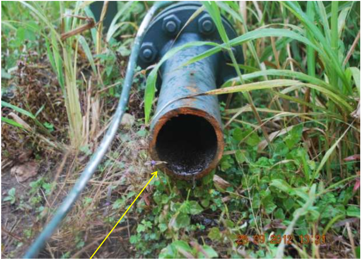
Close-up: Missing Flowline on Uzere Well 12 Flowline at Ezede-Uzere. Picture was taken during Joint Investigation of 25 th Sept. 2012.
