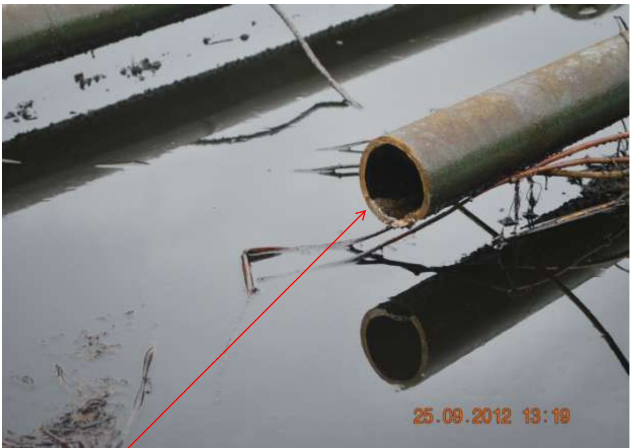
Close-up: Missing Flowline on Uzere Well 12 Flowline at Ezede-Uzere. Picture was taken during Joint Investigation of 25 th Sept. 2012.
