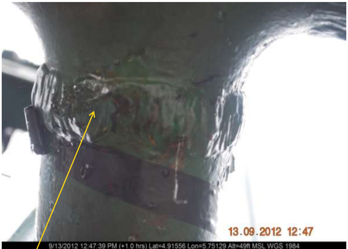
Close-up: Internal corrosion on Opukushi Well 25 at Agbediama. Picture was taken during Joint Investigation of 13 th Sept. 2012
