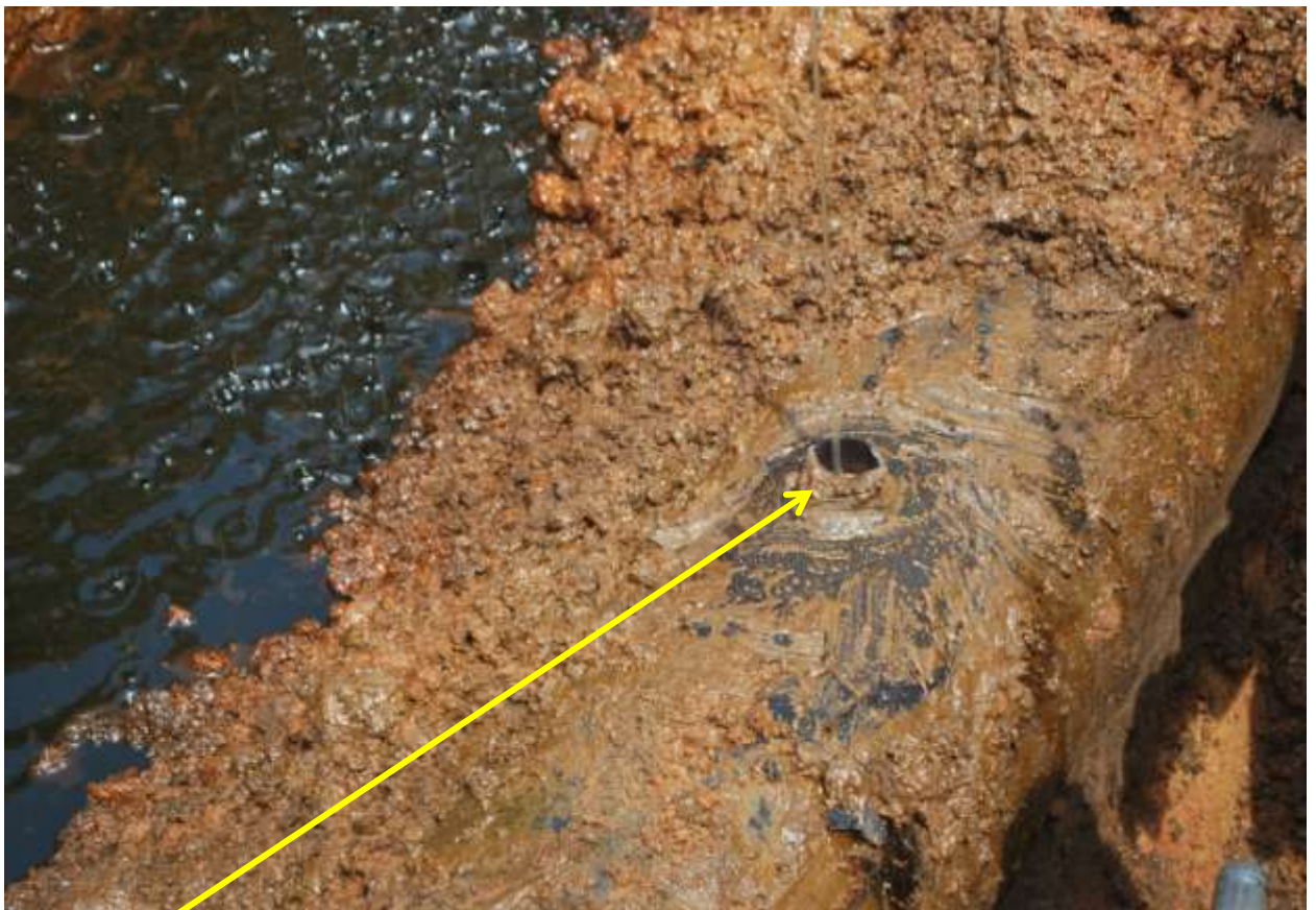
Close-up: Drilled hole on 16" Uzere - Eriemu Trunkline at Iyede. Picture was taken during Joint Investigation of 18th Sept. 2012.
