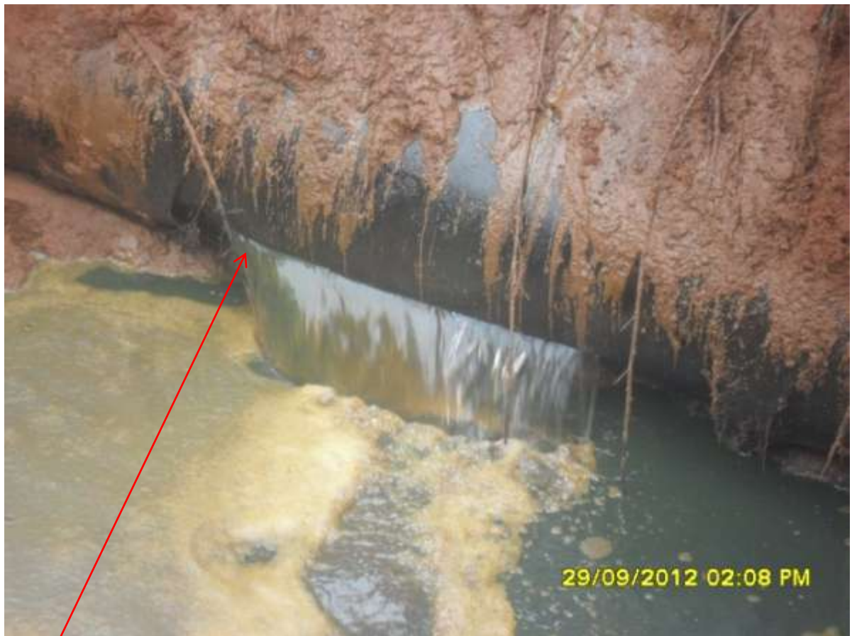
Close-up: Explosive tear on 16'' Egbema-Assa Pipeline At Umudike. Picture was taken during Joint Investigation of 29 th Sept. 2012.
