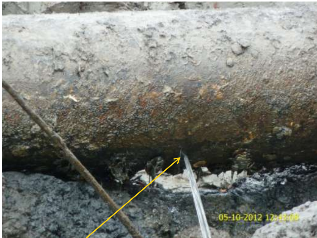
Close up: Spill point due to corrosion on 24" Bomu-Bonny Trans Niger pipeline at Freetown. Picture was taken during Joint Investigation of 5 th October 2012.
