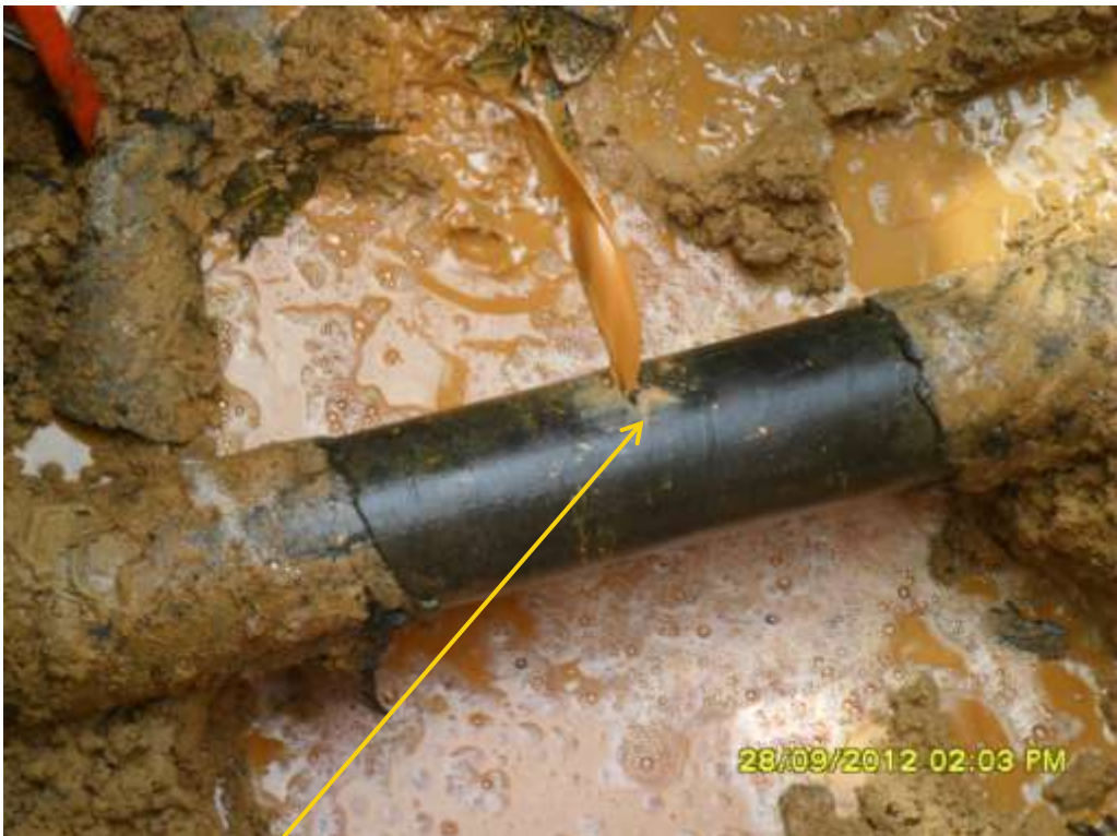
Close up: Hacksaw cut on 4" Obelle-Ibaa pipeline at Ibaa. Picture was taken during Joint Investigation of 28 th September 2012.
