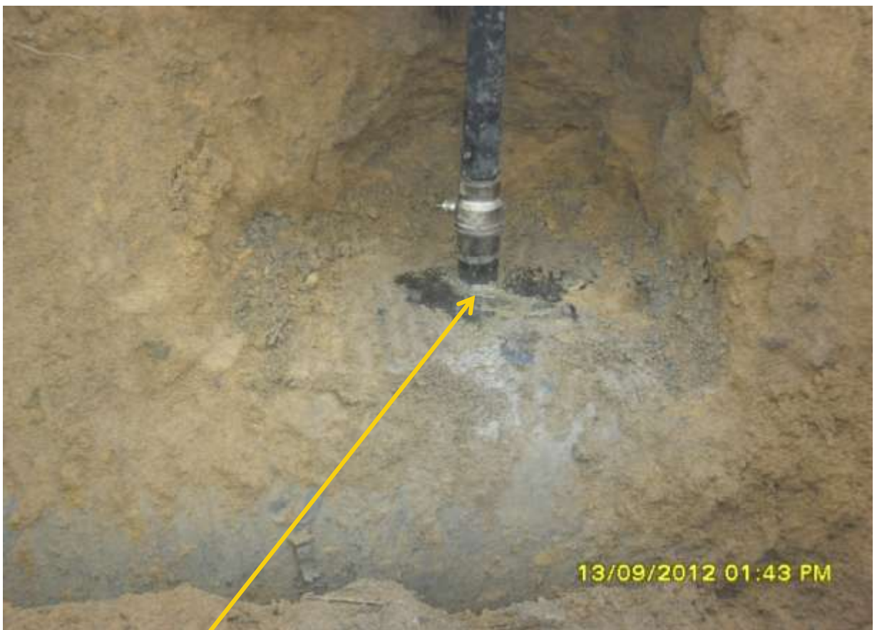
Close-up: Illegal fitting on 28" Nkpoku-Bomu TNP at Gio. Picture was taken during Joint Investigation of 13 th Sept. 2012.
