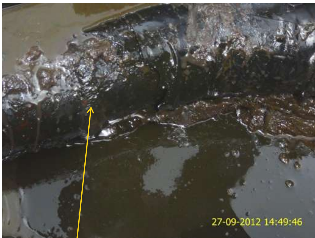
Close up: Failed weld on 4" Santa Barbara Well 11T flowline at Ikegimakiri. Picture was taken during Joint Investigation of 27 th September 2012.
