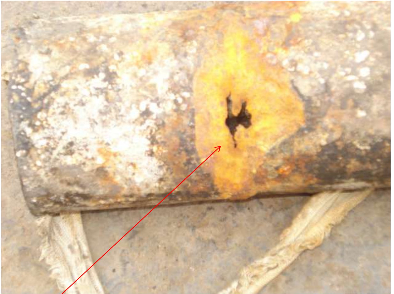
Close-up: Submerged location of corrosion on Bonny Well 2S Flowline at Bonny. Picture was taken after retrieval of failed section.
