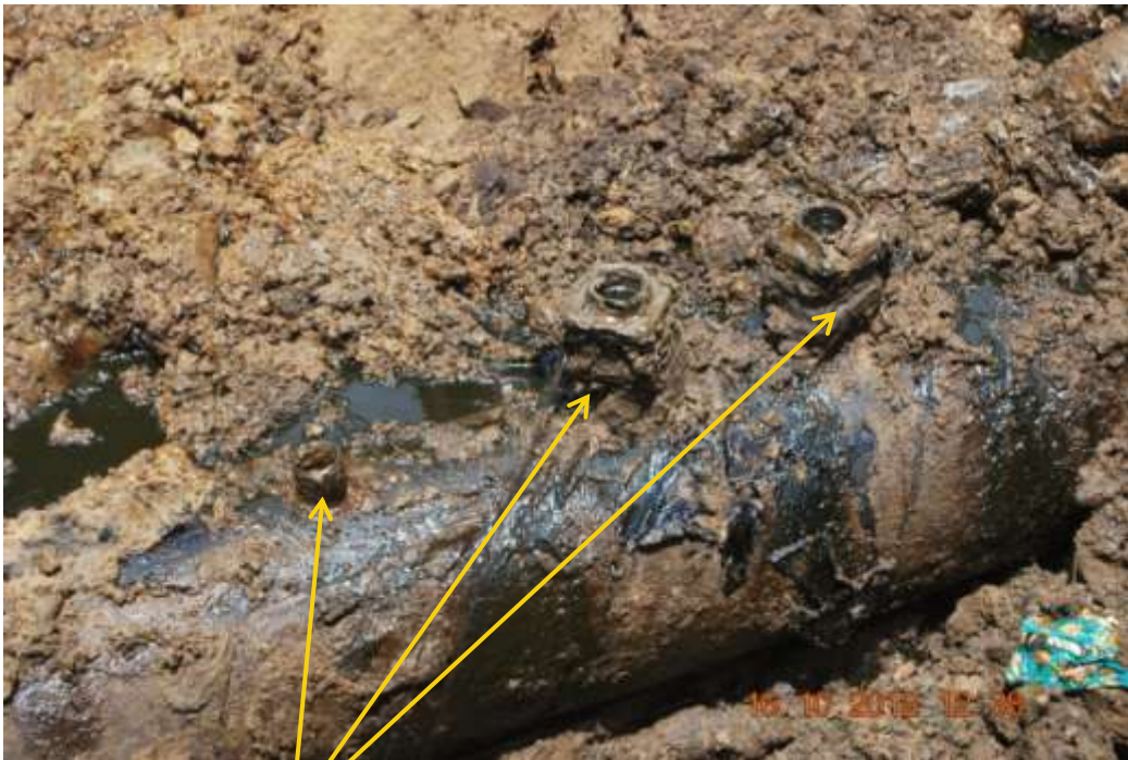
Close up: Illegal fittings on 16" Eriemu-UPS trunkline at Ekiugbo. Picture was taken during Joint Investigation of 16 th October 2012.
