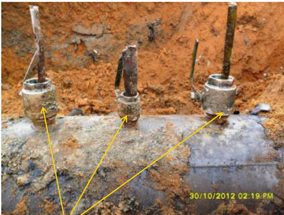
Close up: Illegal fittings on 28" Nkoku-Bomu pipeline at Elenwo. Picture was taken during Joint Investigation of 30 th October 2012.
