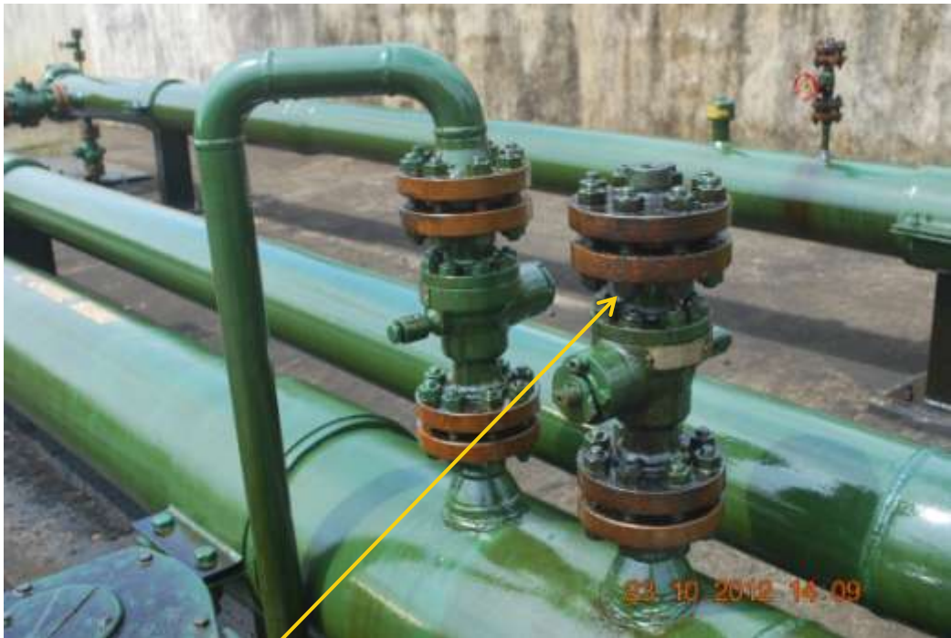
Close up: Leak from vent valve on 12" Afiesere-Eriemu delivery line at Gana. Picture was taken during Joint Investigation of 23 rd October 2012.
