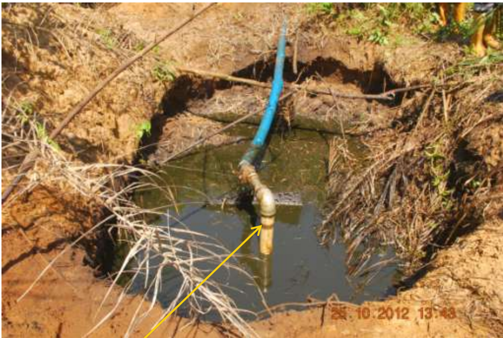
Close up: Illegal fitting on 20" Otumara-Escravos pipeline at Adjudiabo. Picture was taken during Joint Investigation of 25 th September 2012.
