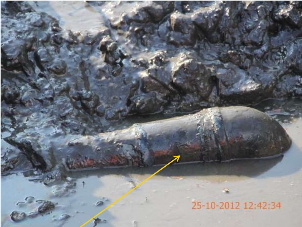
Close up: Illegal fitting on 20" Otumara-Escravos pipeline at Ugboegungun. Picture was taken during Joint Investigation of 25 th September 2012.
