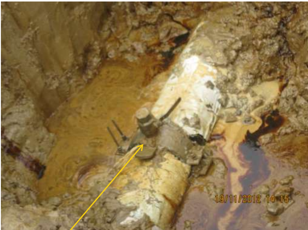
Close up: Illegal fitting on 12" Imo River2 – Oghale pipeline at Uzuaku. Picture was taken during Joint Investigation of 19 th November 2012.
