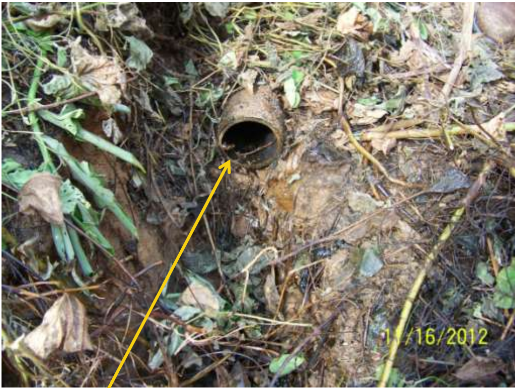
Close up: Cut section on Imo River1 Well18 flowline at Owaza. Picture was taken during Joint Investigation of 16 th November 2012.
