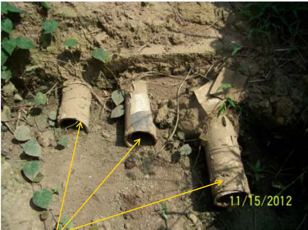
Close up: Cut sections on Obigbo Well28LS flowline at Umuebulu. Picture was taken during Joint Investigation of 15 th November 2012.
