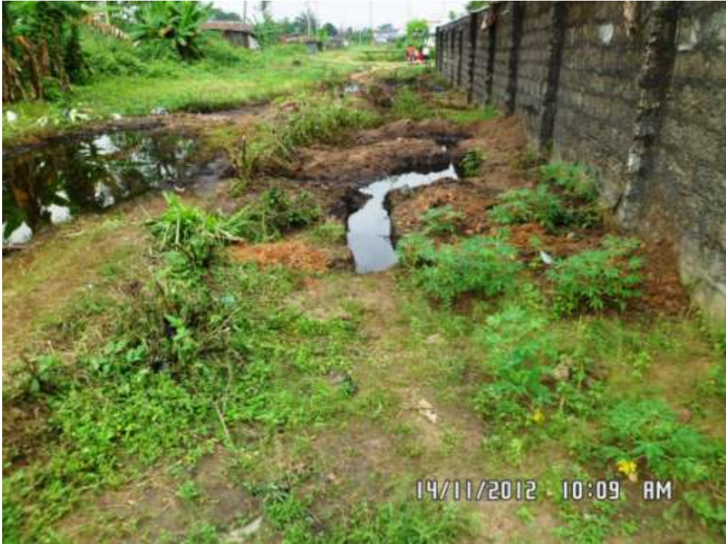
Overview: Part of spill impact on 8" Obigbo North-Komkom pipeline right of way at Umuokolobo. Picture was taken during Joint Investigation of 14 th November 2012.
