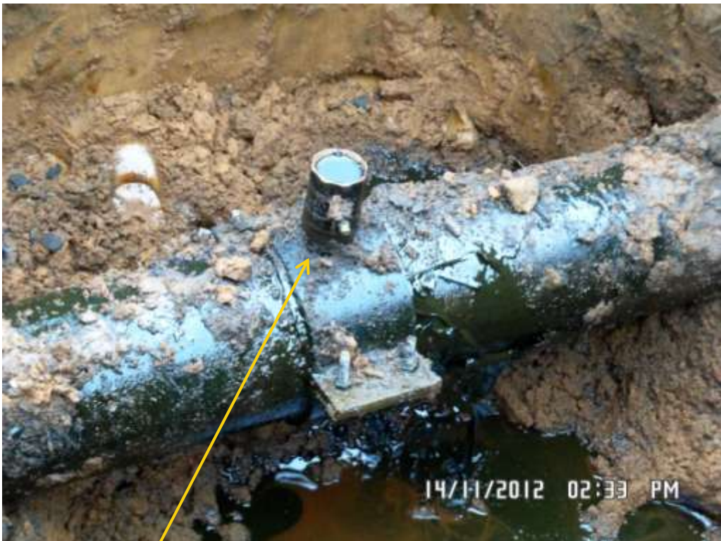
Close up: Illegal fitting on 8" Obigbo North-Komkom pipeline at Umuokolobo. Picture was taken during Joint Investigation of 14 th November 2012.
