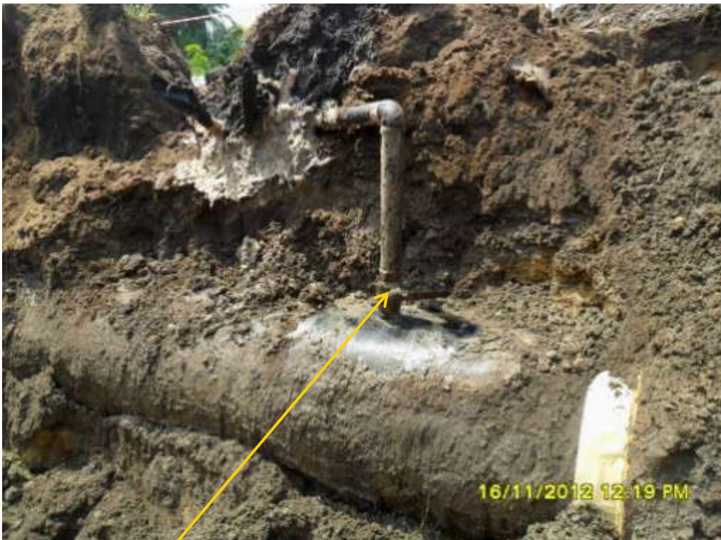
Close up: Illegal fitting on 24" Bomu-Bonny pipeline at Mogho. Picture was taken during Joint Investigation of 16 th November 2012.
