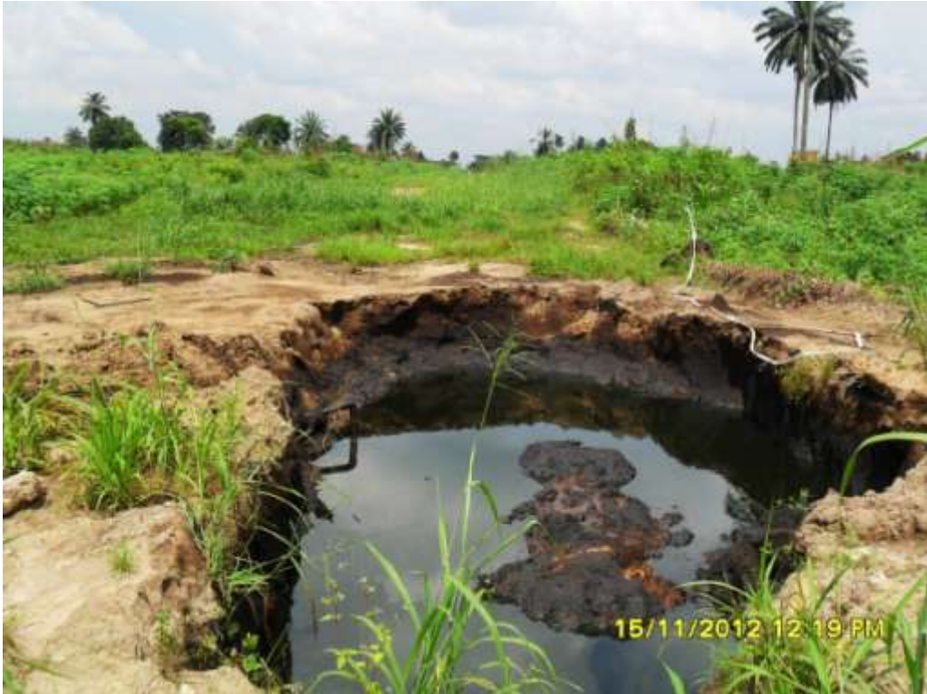
Overview: Part of spill impact on 24" Bomu-Bonny pipeline right of way at Mogho. Picture was taken during Joint Investigation of 15 th November 2012.
