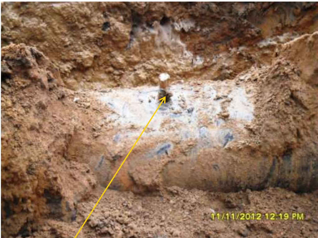
Close up: Illegal fitting on 28" Nkpoku-Bomu pipeline at Gio. Picture was taken during Joint Investigation of 11 th November 2012.
