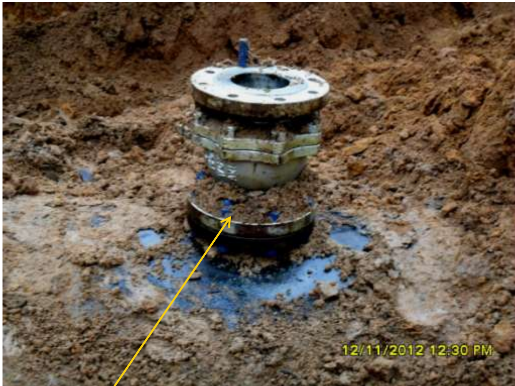
Close up: Illegal fitting on 28" Nkpoku-Bomu pipeline at Gio. Picture was taken during Joint Investigation of 12 th November 2012.
