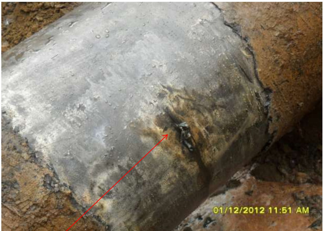
Close-up: Hacksaw cut on 24 inch Nkpoku – Bomu Pipeline at Egbalor. Picture was taken during Joint Investigation of 1 st Dec. 2012.
