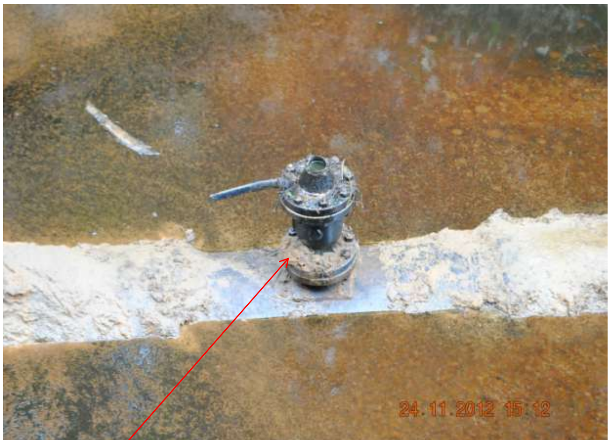
Close-up: Illegal fitting on 20 inch Otumara - Escravos Pipeline at Escravos. Picture was taken during Joint Investigation of 24 th Nov. 2012.
