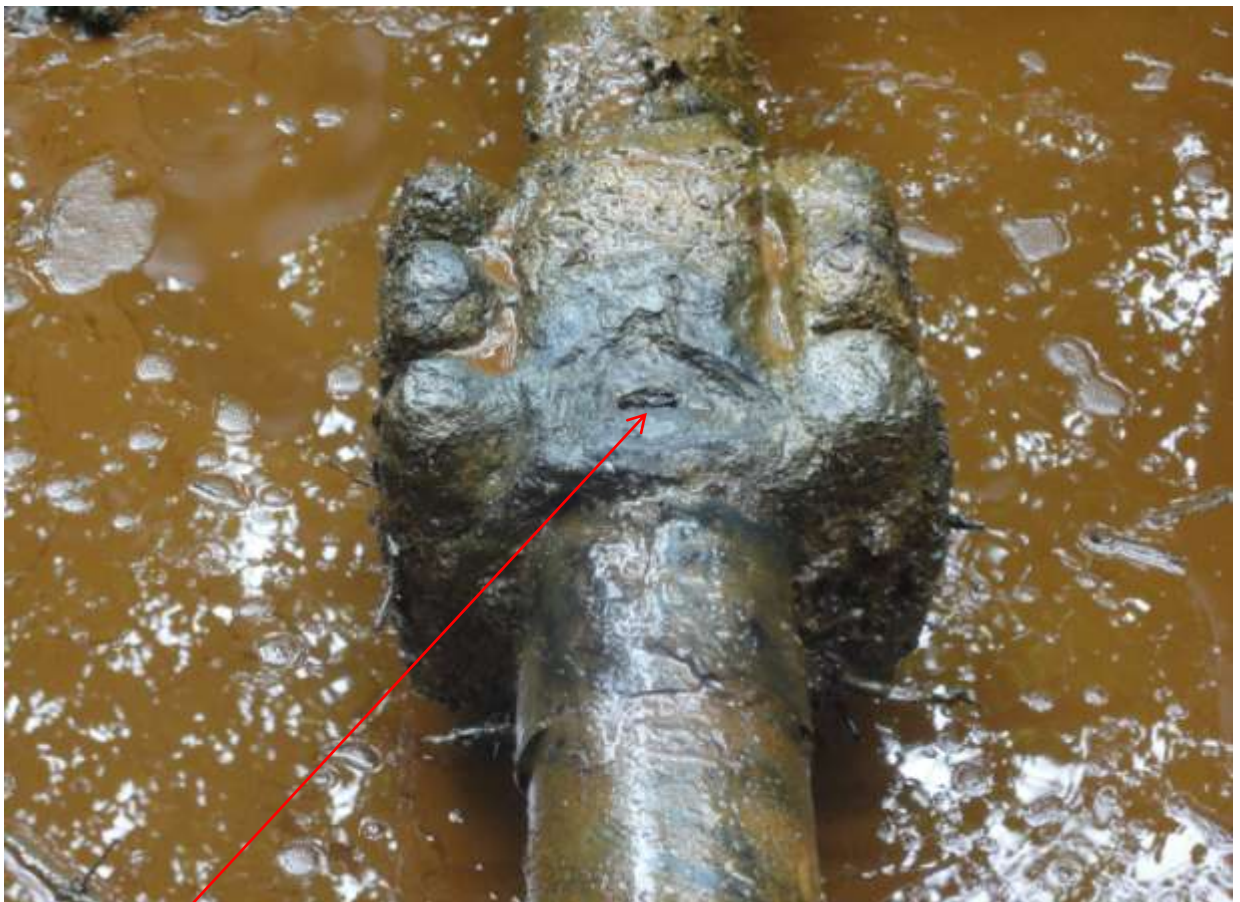
Close-up: Failed Clamp on Cawthorne Channel 2 Well 28T at Owame-Ama Okpoama. Picture was taken during Joint Investigation of 28 th Nov. 2012.
