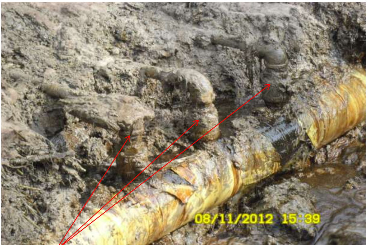
Close-up: Illegal fittings on 12 inch Imo River1 and 2- Ogale Pipeline at Komkom. Picture was taken during Joint Investigation of 8th Nov. 2012
