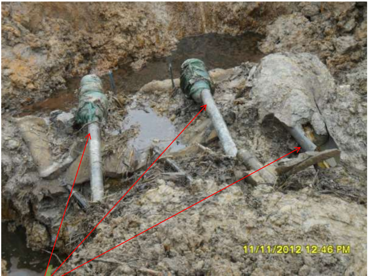
Close-up: Illegal fittings on 12 inch Imo River1 and 2- Ogale Pipeline at Komkom. Picture was taken during Joint Investigation of 11th Nov. 2012
