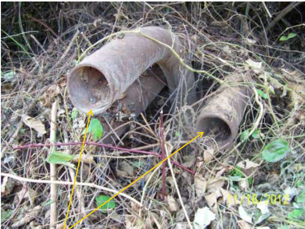
Close up: Cut sections on Imo River1 Well25S flowline at Owaza. Picture was taken during Joint Investigation of 16 th November 2012.
