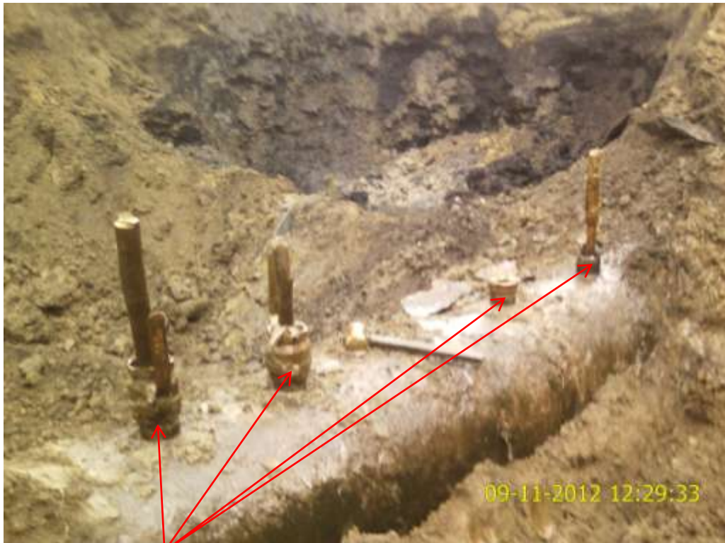
Close up: Illegal fittings on 24" Nkpoku-Bomu pipeline at Biara. Picture was taken during Joint Investigation of 9 th November 2012.
