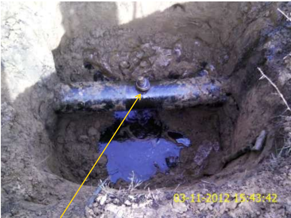
Close up: Illegal fitting on 8" Obigbo North – Eelenwa pipeline at Umusia. Picture was taken during Joint Investigation of 3 rd November 2012.
